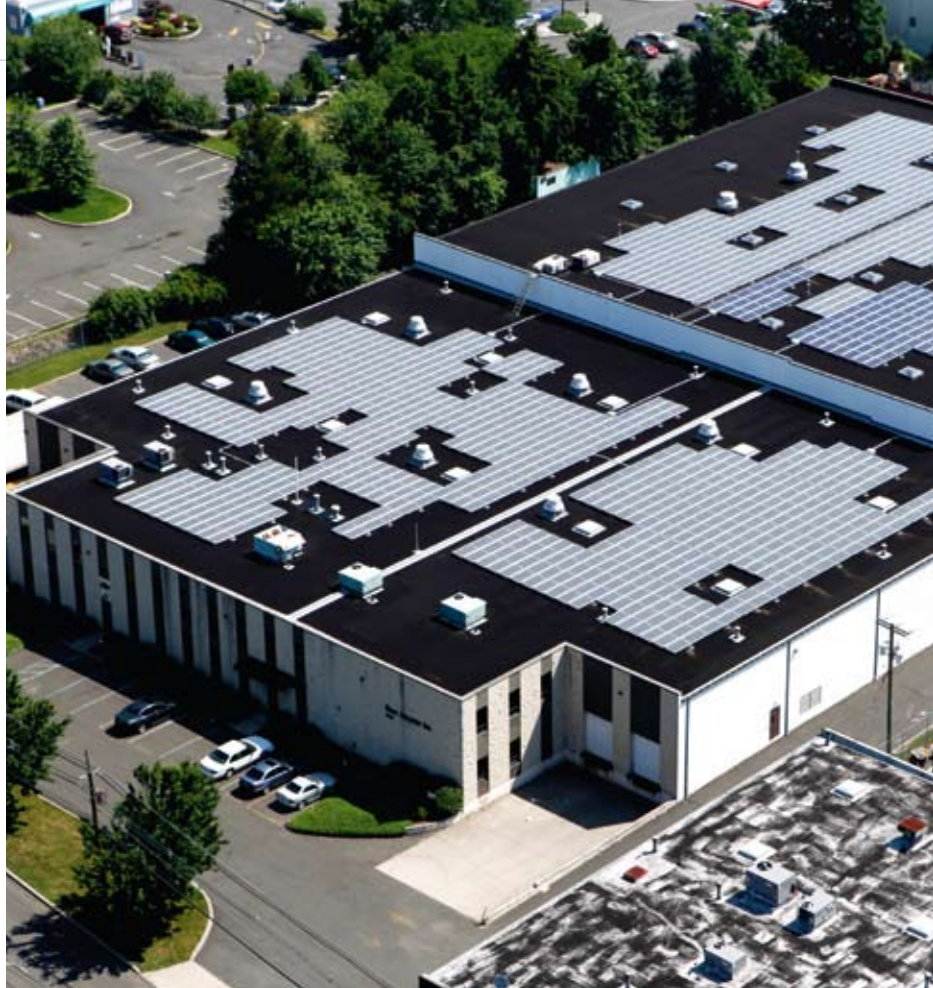
This large commercial system in New Jersey was installed by SunPower dealer GeoGenix.
